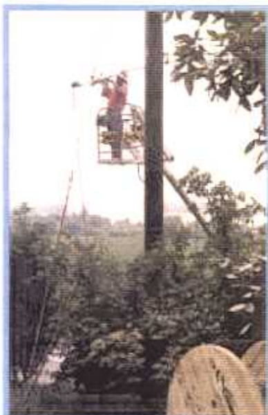
Installation of overhead fiber optic cable came as a response to public demand for bundled services in Muscatine, Iowa.
